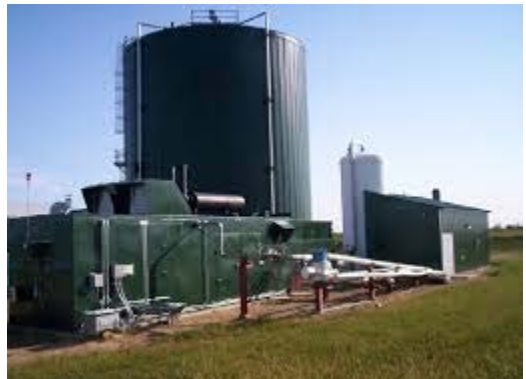
Complete mix digester at Wild Rose Dairy in Webster Township, WI, uses manure from 880 cows and food waste as fuel to produce 775 kW of electricity.
